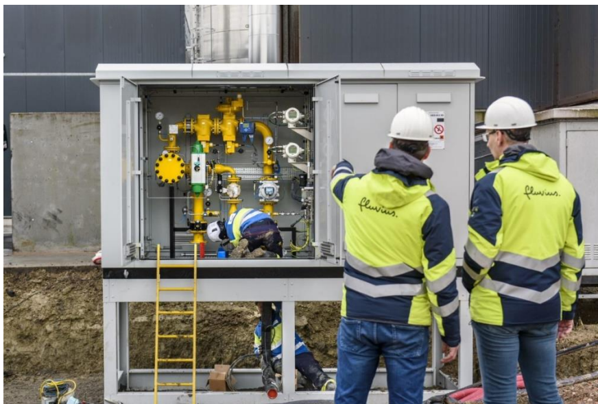
The biomethane injection installation in Ypres
