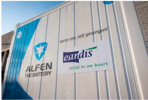
battery for energy storage (Lokeren)
